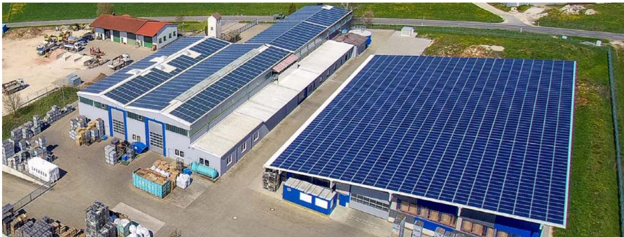
FIGURE 96. PHOTOVOLTAIC INSTALLATIONS ON THE ROOF OF THE HP-T HÖGLMEIER POLYMER-TECH GMBH IN BAVARIA
